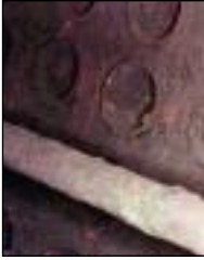
This image shows oxygen pitting in a boiler drum that was given inadequate layup protection. Courtesy: EPRI
