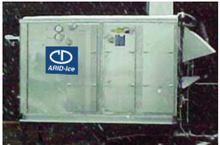
Curbside installation rated at 5,500 SCFM
