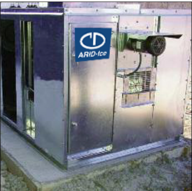
Outdoor slab installation rated at 3,000 SCFM.
